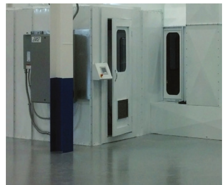
Control panel beside the booth door.
