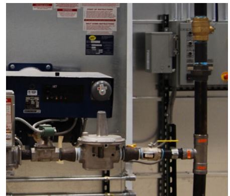
Burner and gas train on an air make-up unit.
