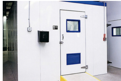
AFC paint mixing room.
