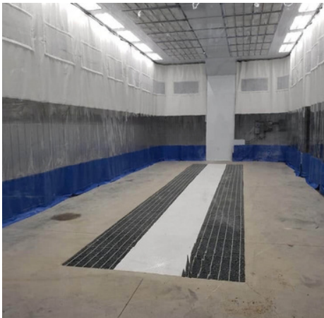
AFC work station with curtains and floor grating.
