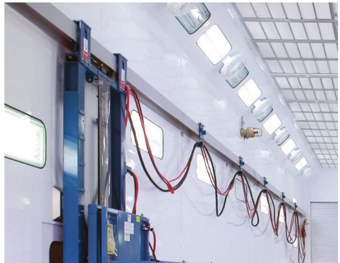
Painter lift and light fixtures inside a booth.
