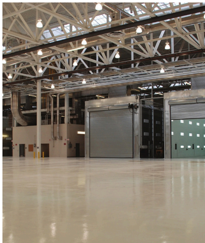
Spray booths on a production floor.
