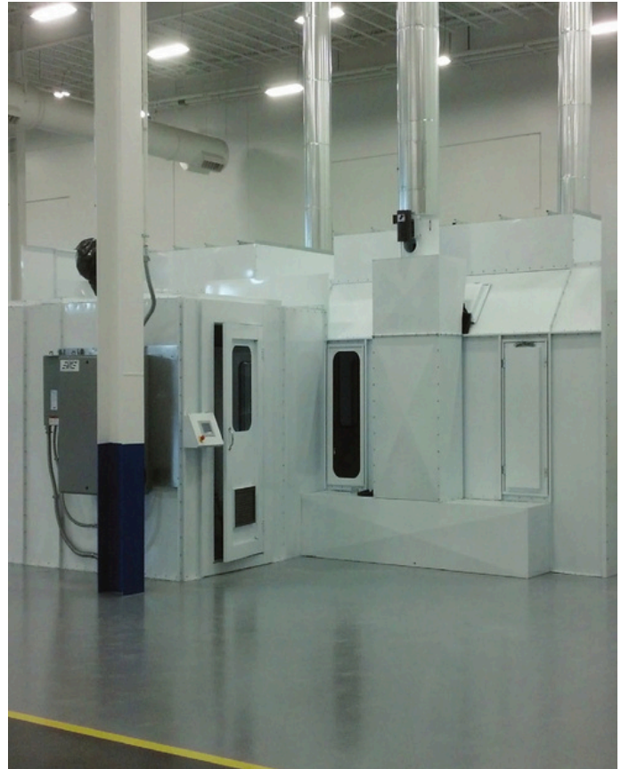
AFC booth and ductwork on the shop floor.
